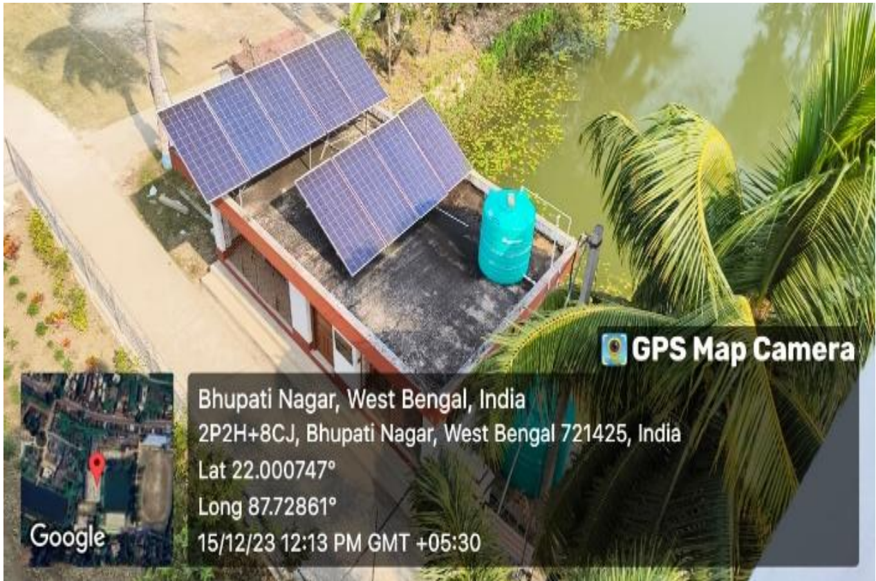
Solar Panel installed on the roof of the pond water purifier house
